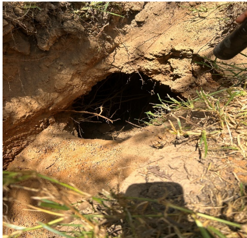
Sinkhole caused by Wastewater Trunk Main
