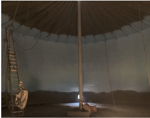
Ragley 1,500,000 Million Gallon Tank
