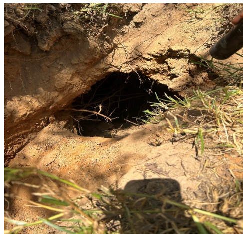
Sinkhole caused by Wastewater Trunk Main
